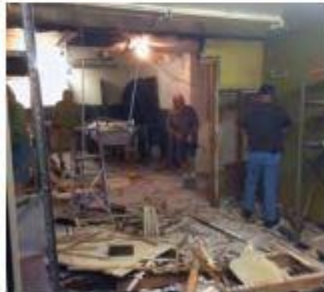
The DAW crew knee-deep in demolition, knocking down walls and moving electrical and plumbing, to make smaller units into a larger, more functional space.
