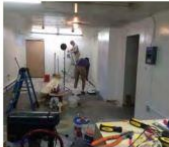
Reconstruction involved updating and adding light fixtures, drywall, and paint, as well as filling, leveling, and sealing the floor.
